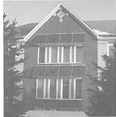
Photovoltaic panels installed on the InfoCentre of the Canadian Centre for Housing Technology
