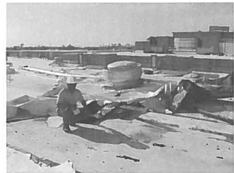
An IRC researcher surveys roof damage caused by Hurricane Katrina
