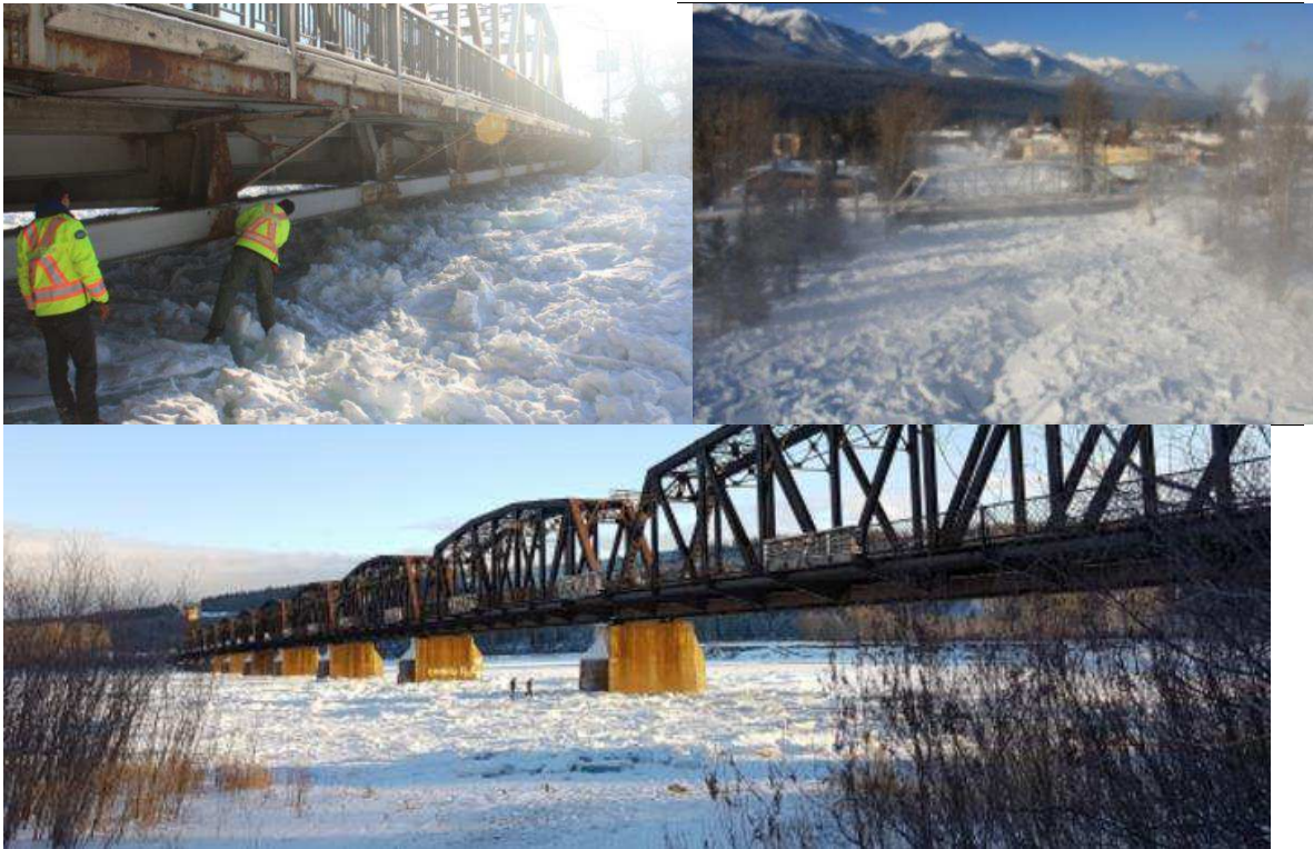
Figure 2. Top left and right) Ice reaching the superstructure of a bridge located in Golden, across the Kicking Horse River on Highway 95. 2 Bottom) Ice jam in Prince George on the railway bridge at the confluence of the Fraser River and the Nechako River. 3
