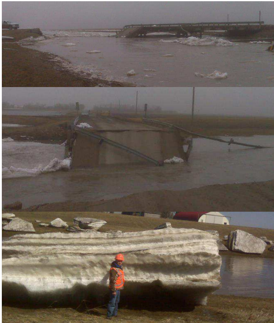
Figure 6. Collapse, due to ice loading, of a bridge located on Tobacco Creek on PR 332 (MB). Courtesy of Manitoba Infrastructure and Transportation.
