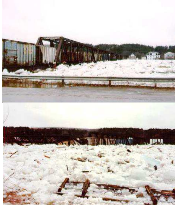
Figure 7. Top) Ice jam at a railway bridges in New Brunswick. Bottom) Collapsed bridge under ice forces. Images from the NB River Ice Manual.
