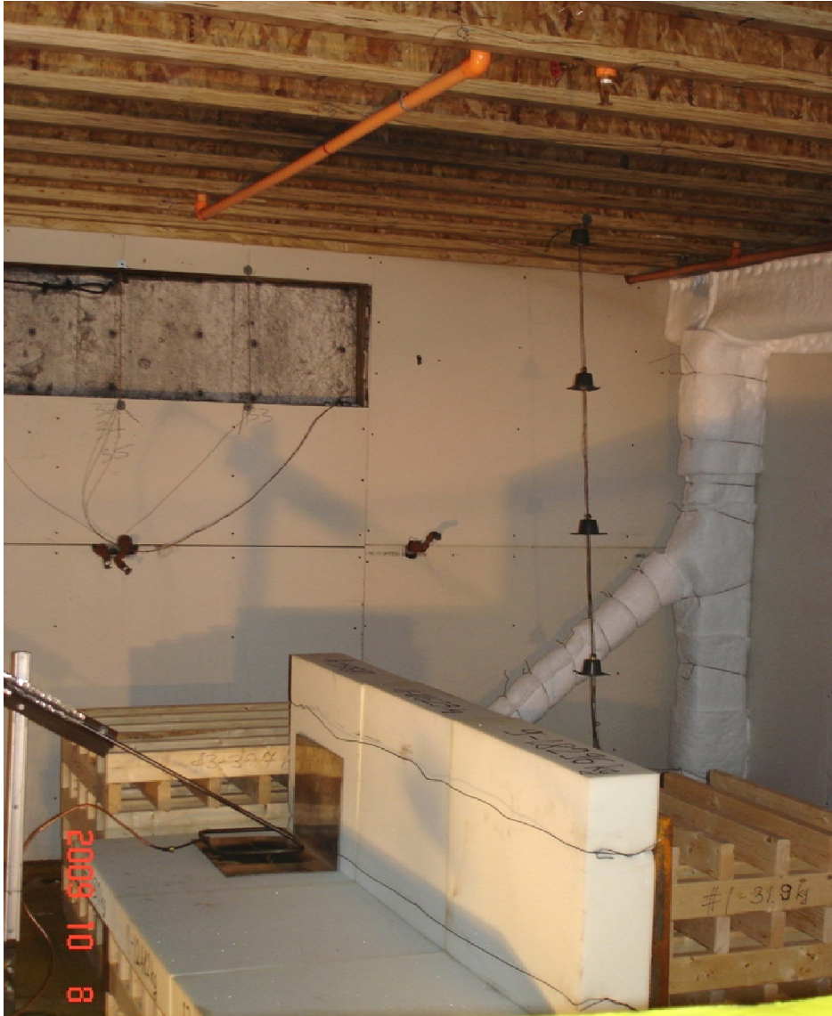
Figure 73. Sprinkler and CPVC piping relative to exposed wood I-joists and fuel (Test PF-03B)
