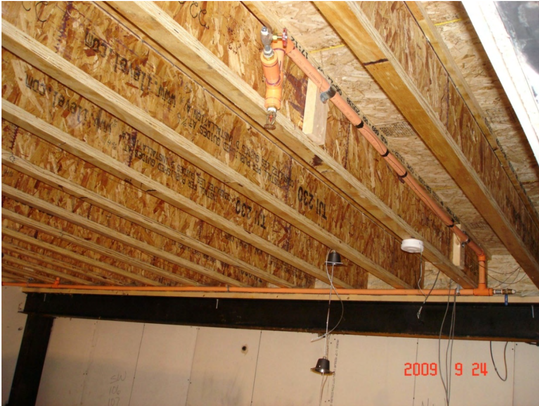
Figure 63. Sprinkler and CPVC piping installation with exposed wood I-joists in Test PF-03
