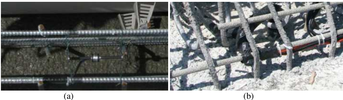
Figure 5. Instrumentation of the barrier: (a) VWSG (EM5) embedded in concrete; (b) Thermometers (TH-T) attached to the reinforcing bars
