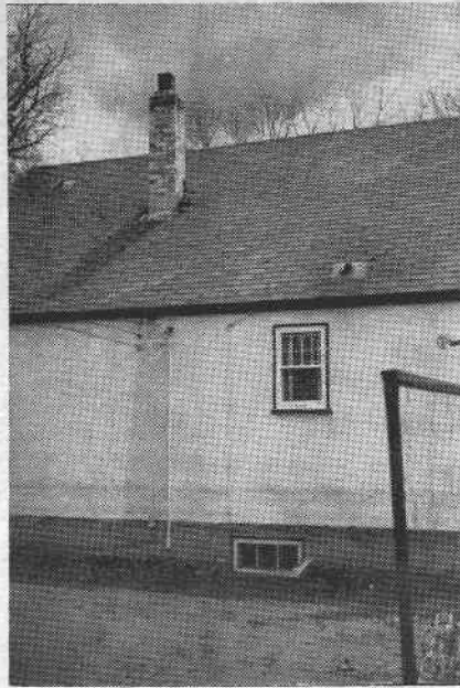
CHIMNEY lifted 3 inches by differential movement between foundation walls and chimney footings.
