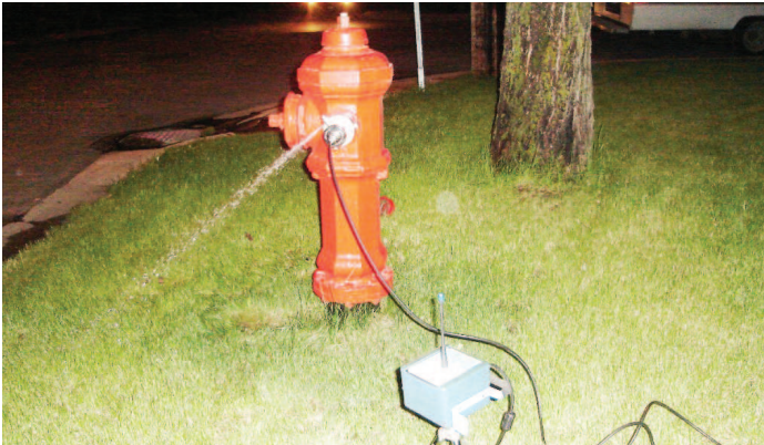
Figure 4. Hydrophone connected to a fire hydrant
