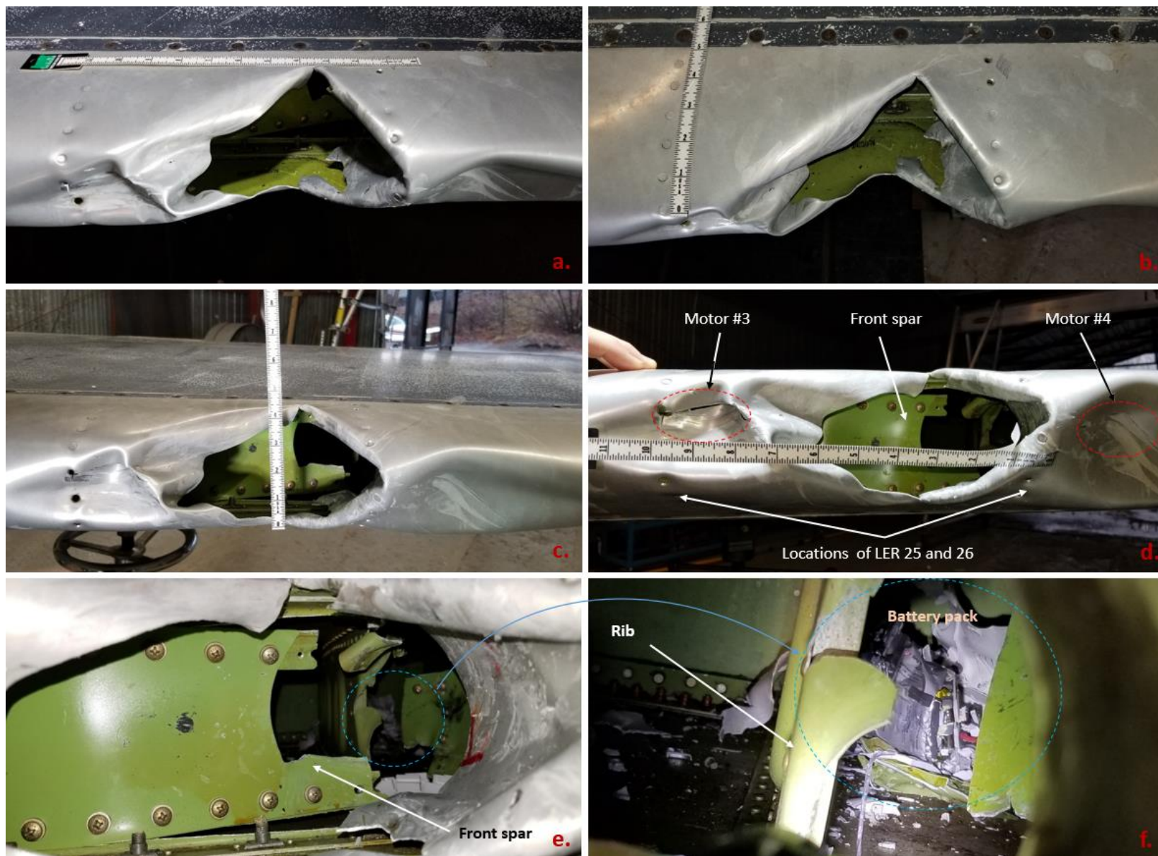
Figure 14: Pictures of damaged HS leading edge (Test #1: HS-T1)
