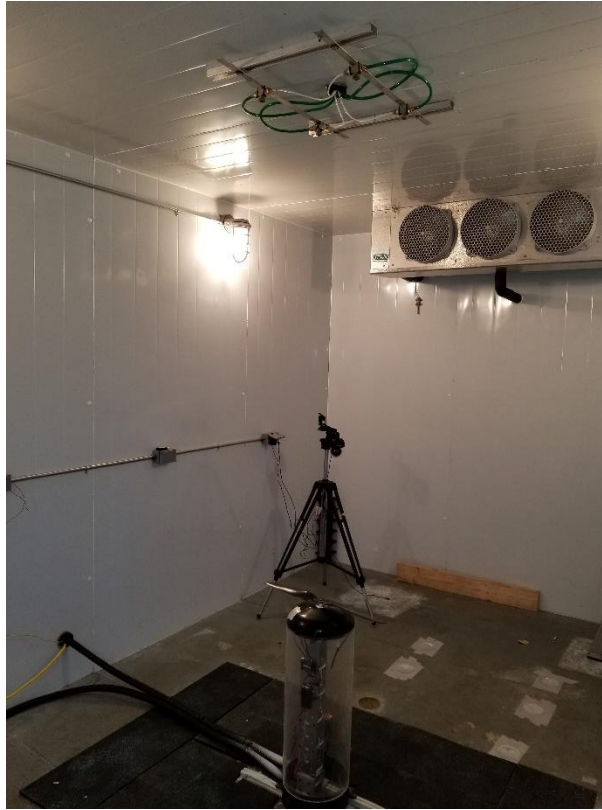
Figure 41: Spray system and rotor thrust stand installed in cold room
