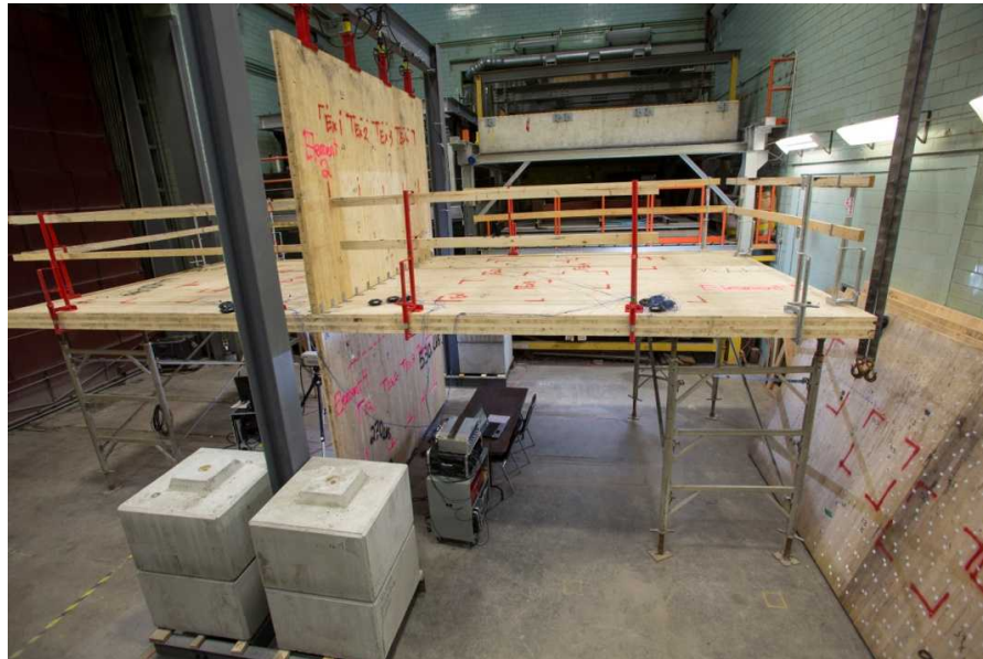
Figure A.4 - 4: CLT floor-wall junction mock-up with loading frame and measurement system
