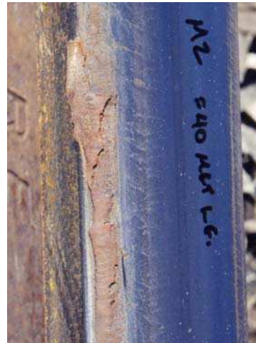
A) gauge-corner collapse in a dry environment
