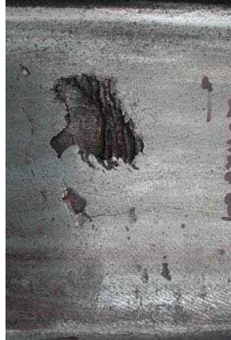
H) Continued propagation of cracks into the wheel surface leads to tread shelling.
