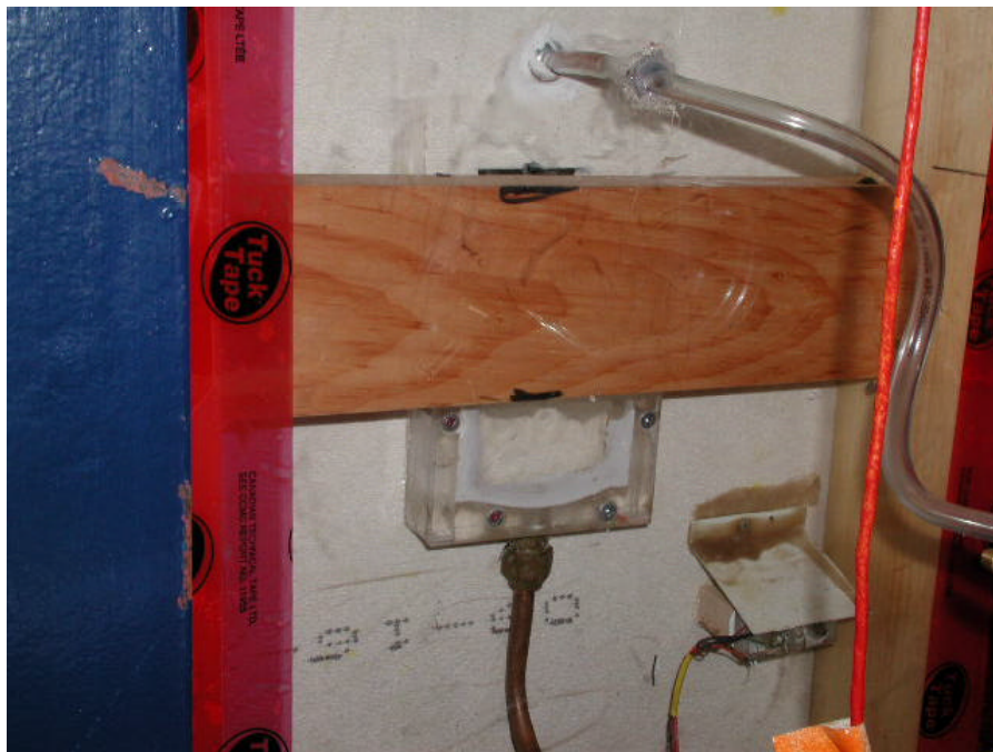
Figure 4.6 – EIFS WA-8 : Water entering through deficiency above electrical outlet but draining between gypsum board and EPS insulation.
