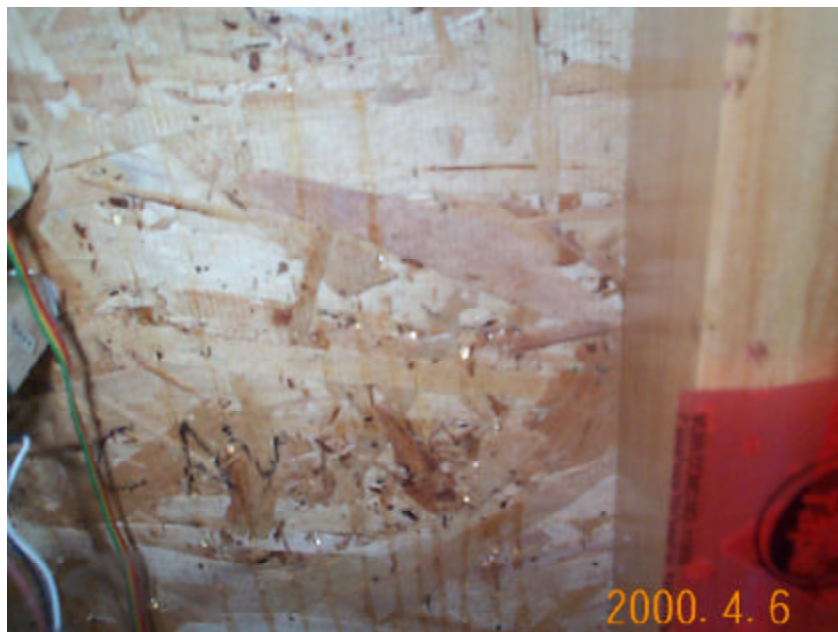
Figure 4.12 – EIFS WA-6 Stage 6 (sealant removed and backing rod in place): Cavity beneath ventilation duct. Water coming through pores in sheathing at the start of test – continued throughout Stage 6 and thereafter in Stage 7.
