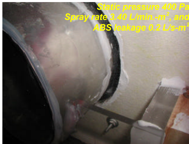
Figure 4.7 – EIFS WA-8 : Stage 7 - at test initiation, water coming through deficiency above ventilation duct and slowly draining between glass mat gypsum board and insulation
