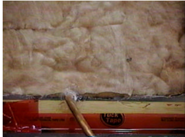
Figure B.50 - Stud cavity at bottom plate after 20 minutes of water accumulation
