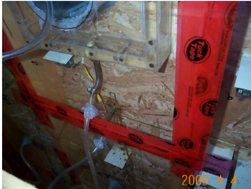
Figure 4.11 – EIFS WA-6 : Water coming through deficiency above ventilation duct and between top and bottom sheathing boards (Stage 5- sealant and backing rod in place). Conditions - Static pressure difference: 300 Pa; Spray rate: 3.4 L/min.-m 2 ; Air Barrier System Leakage: 0.2 L/s-m 2
