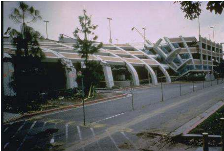
Figure B.13: Extreme example of ductility in concrete, 1994 Northridge earthquake ( http://welldesignedfaith.net/2014/09/12/of-moment-frames-and-church-hymns/ )
