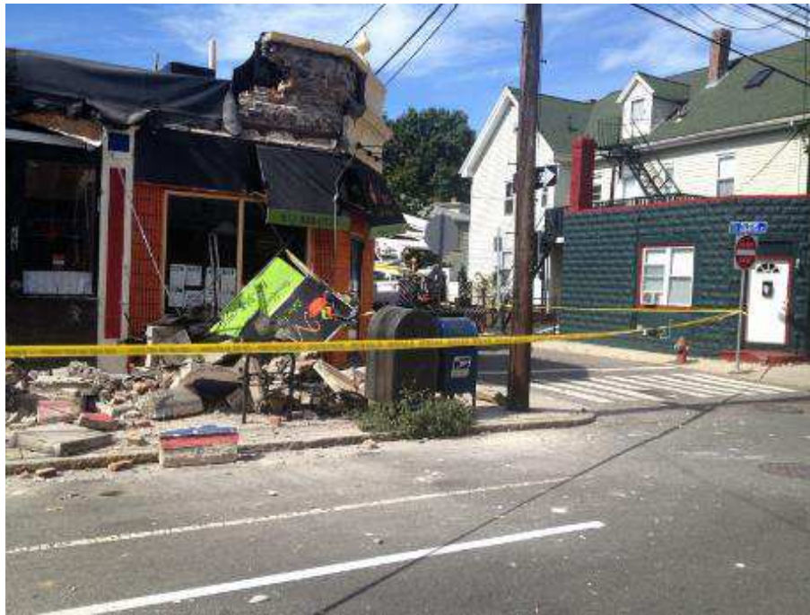
Figure B.30: An example of parapet damage
