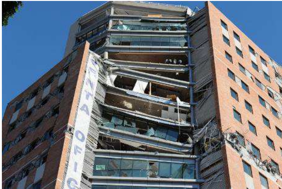
Figure B.15: Shear wall damage ( http://www.reidmiddleton.com/reidourblog/earthquake-reconnaissance-trip-chile/ )
