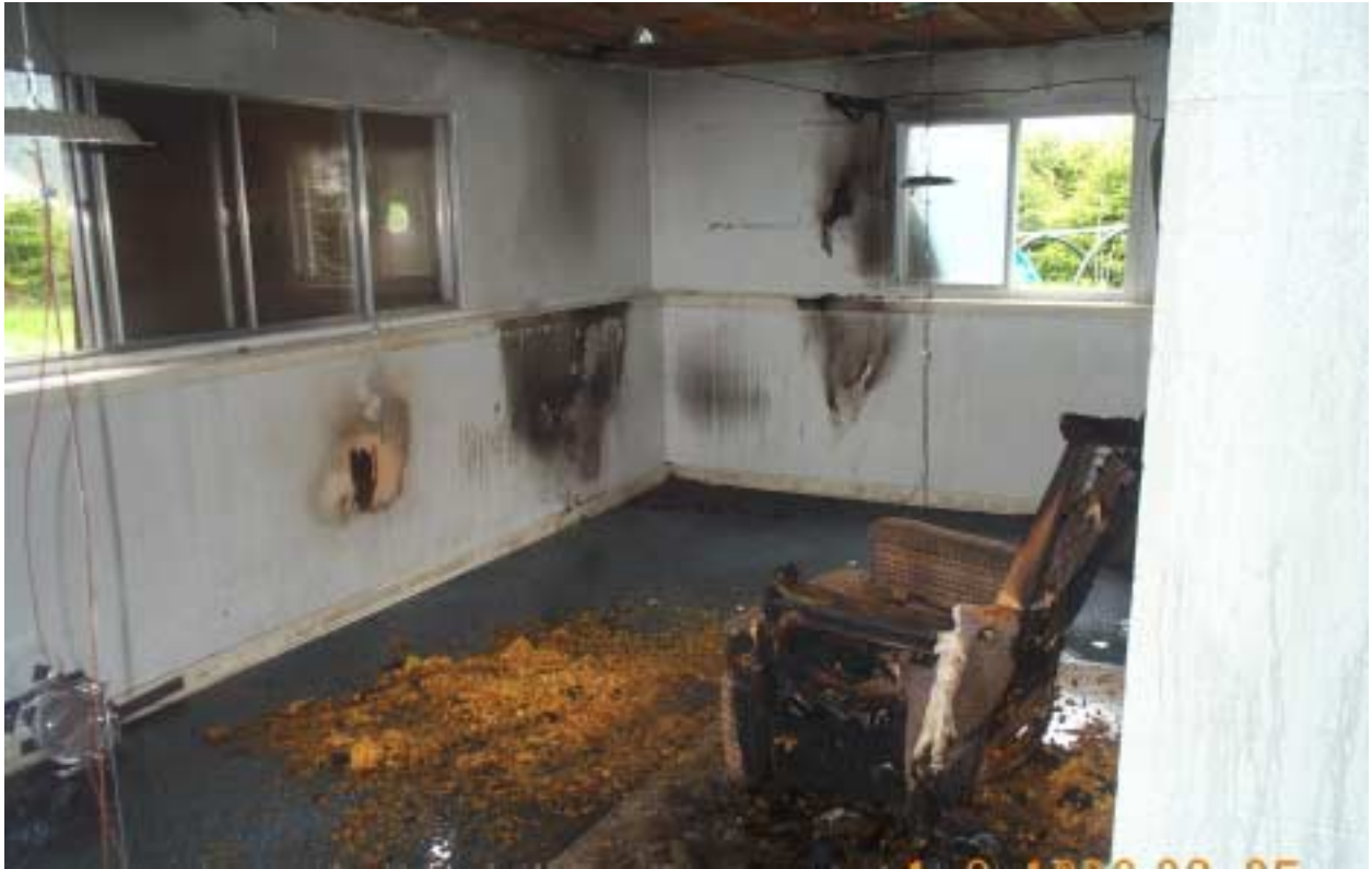
Figure 16. Photograph of the recreation room after Test 2.
