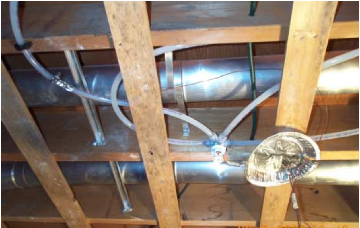
Figure 6. Pipes and fittings on open wood joists in recreation room.
