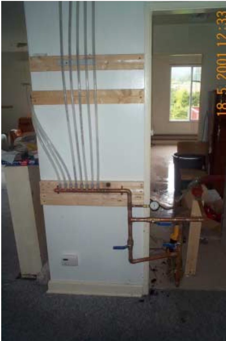
Figure 4. Sprinkler water supply and system manifold.
