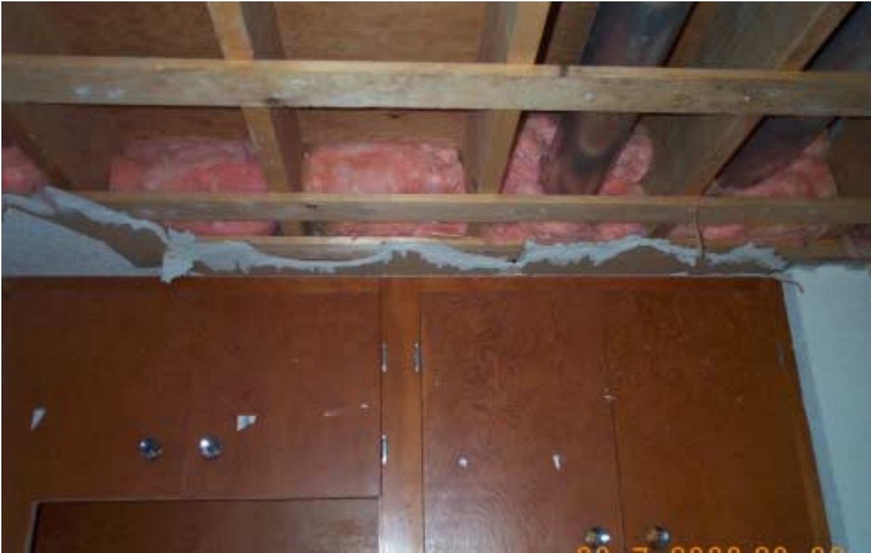
Figure 3. Recreation room ceiling torn down to expose wood joists.
