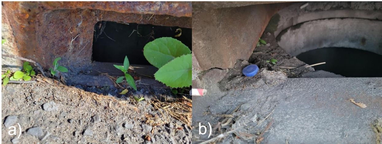
Figure 14. Curb mounted inlets installed in the City of Ottawa; a) S22 and b) S28
