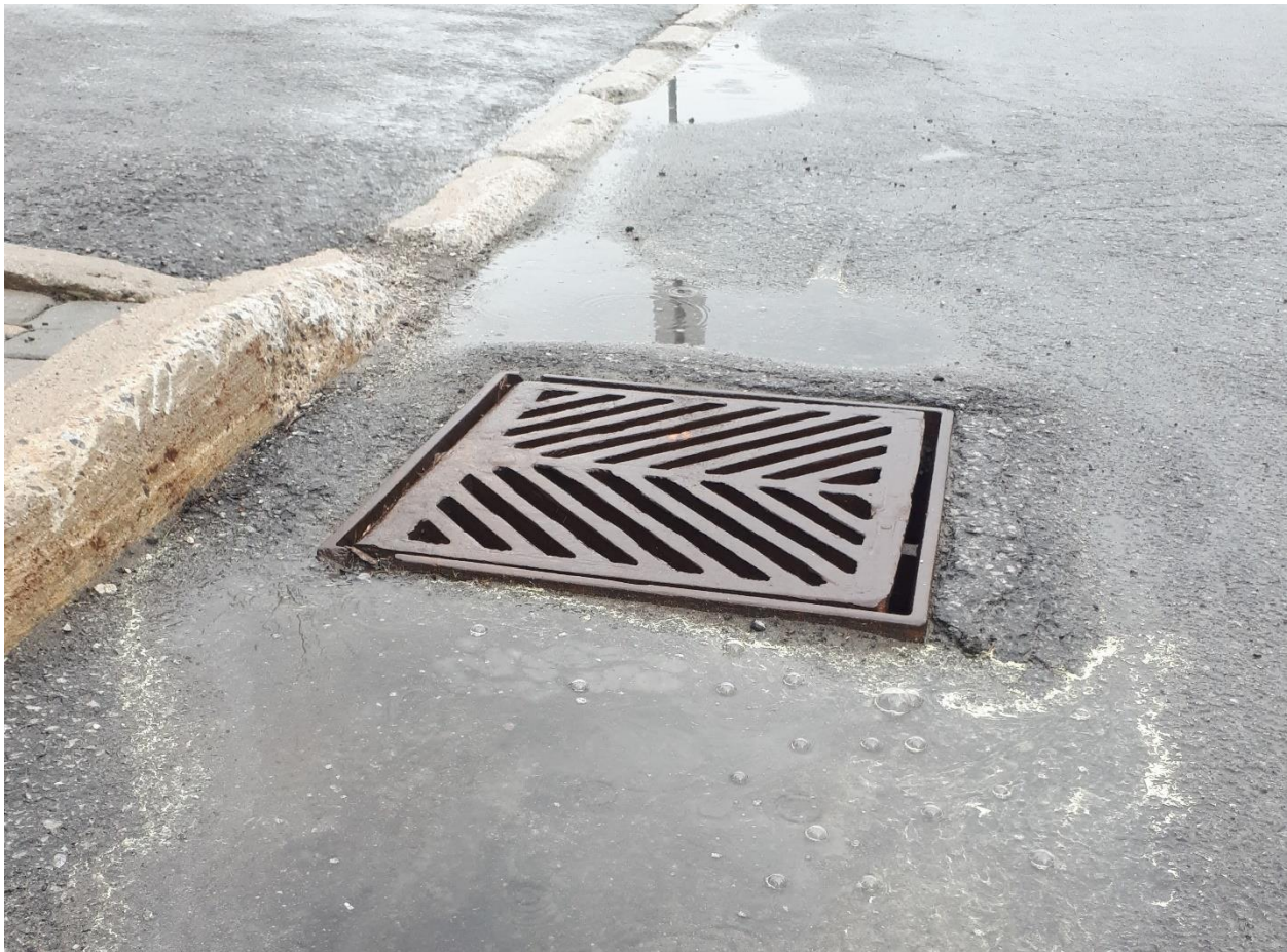
Figure 22. Typical catch basin cover in a roadway
