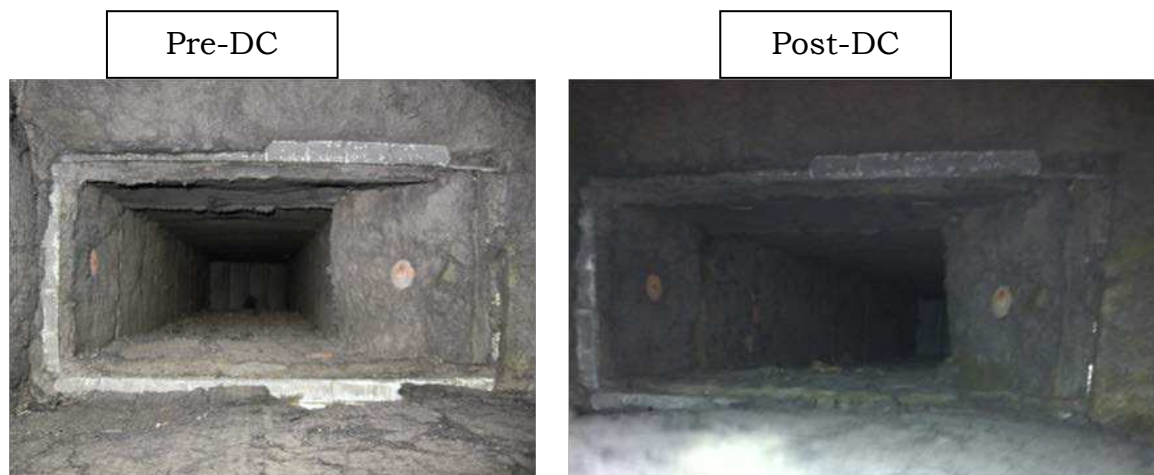
Figure 1 Visual inspection of supply air duct cleanliness pre-& post DC.
