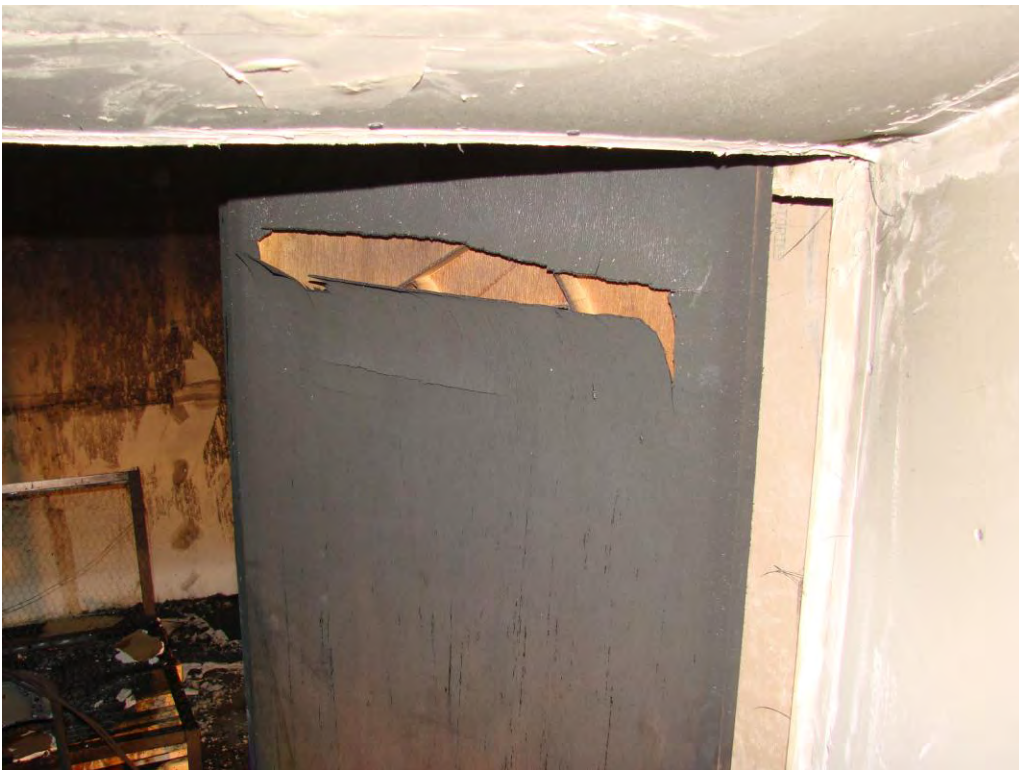
Figure 24. Door to fire compartment after Test 7.
