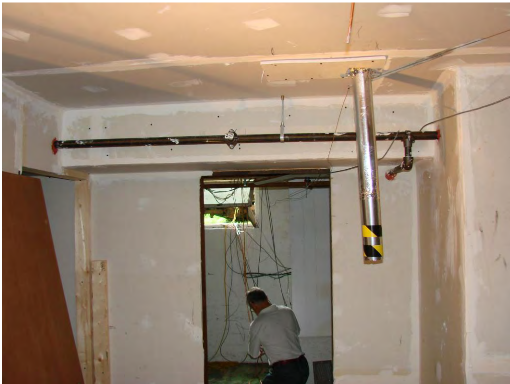
Figure 21. Location of North sprinkler in fire compartment.
