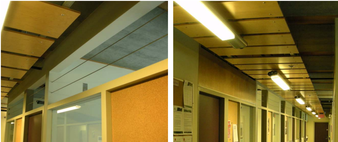
Figure 8. Gaps above doors in Building Q (left), and remedial measure for acoustic concerns (right).
