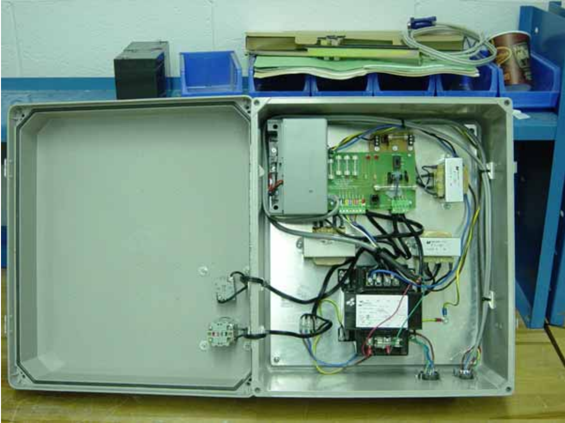
Figure 4. Power Enclosure (Inside).
