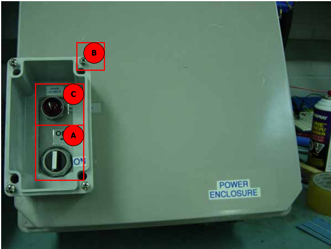
Figure 3. Power Enclosure Main Switch
