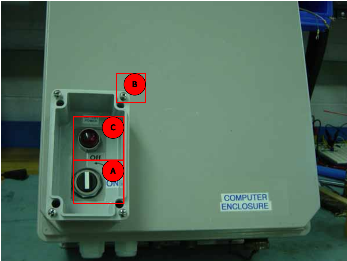
Figure 6. Battery UPS Switch.
