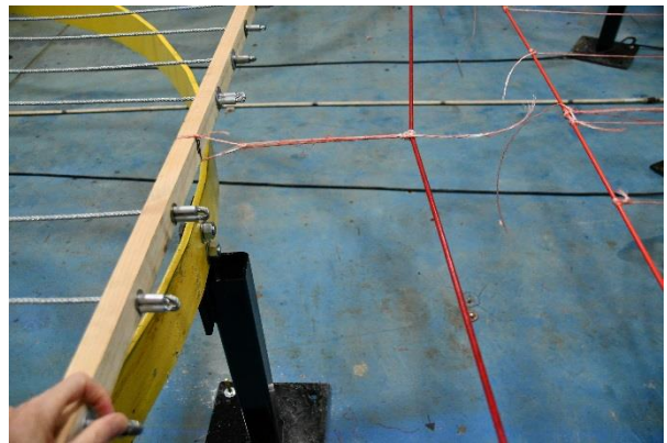
Figure 58: Close-up of reinforcement layout – with W4 again. The red lines were used to apply a tension. The wood onto which are attached the reinforcement cables is tied to that line with plastic cables.
