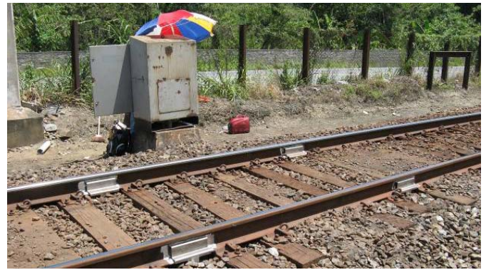
Figure 7 – View of L/V system
