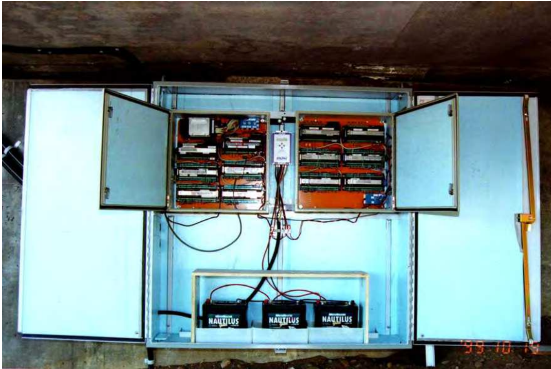
Fig. 3 – Data logging system installed underneath bridge deck
