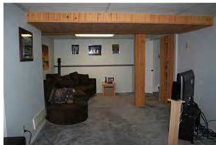
Figure 15. Combustible (wood) ceiling finish
