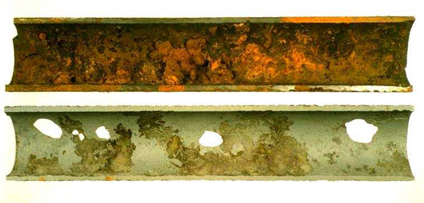
Figure 2. Pipe held water under pressure but found to be totally corroded (source: PDL).
