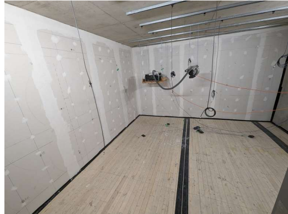
Figure 3: Photo from one of the lower rooms showing the CLT ceiling and the lightweight walls
