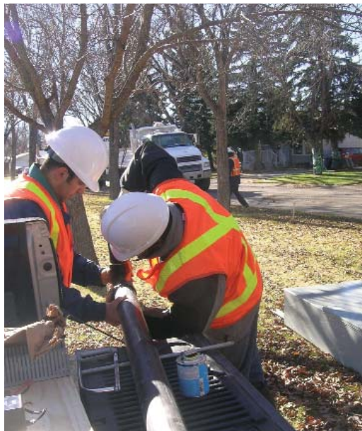
An NRC researcher and a consulting engineer attach gauges to a water pipe
