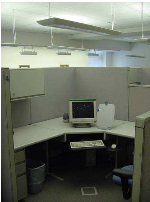
Figure 2. Typical cubicle configuration with single dimmable direct / indirect luminaire centred above and wall washing luminaires in the background.
