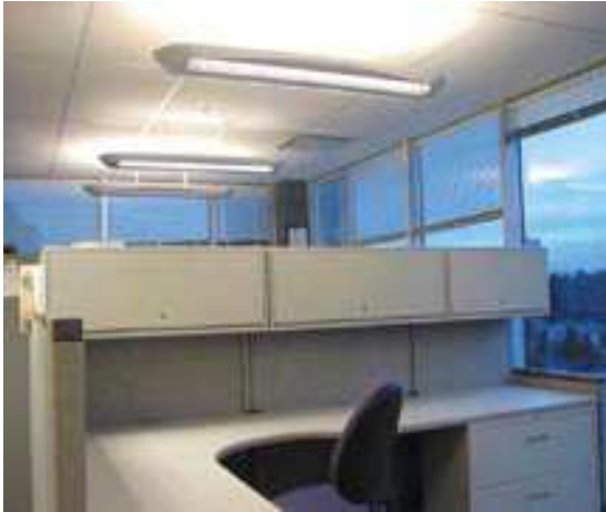
Fig. 2 Typical installation of the luminaires and the window shading.
