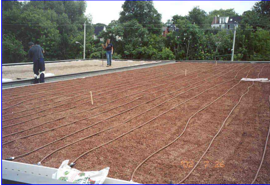
Figure 1: Growing Medium and Irrigation System Being Installed on the Roof of the Eastview Neighbourhood Community Centre
