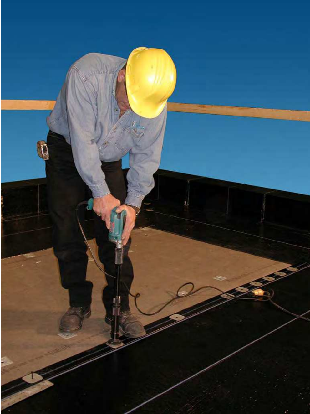
This photo depicts the mechanical attachment of a modified bituminous (mod-bit) system
