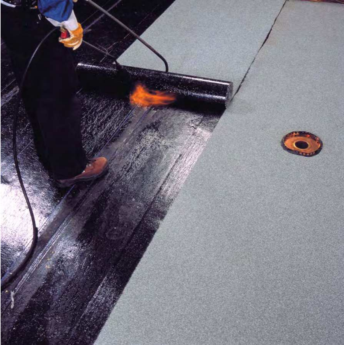
The above photo illustrates the application of cap sheet torching on a two-ply modified bituminous system.
