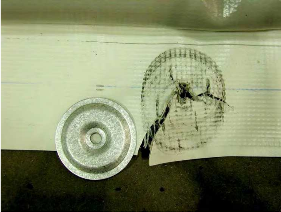
Membrane tear underneath the fastener plate due to lack of clamping force.
