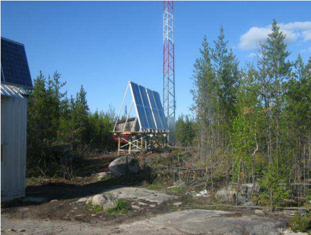
Figure 3: Photo of the solar-powered cellular tower and radio equipment erected in Summer 2008 at Koocheching First Nation, Ontario (photo from the K-Net Media archive http://media.knet.ca ).
