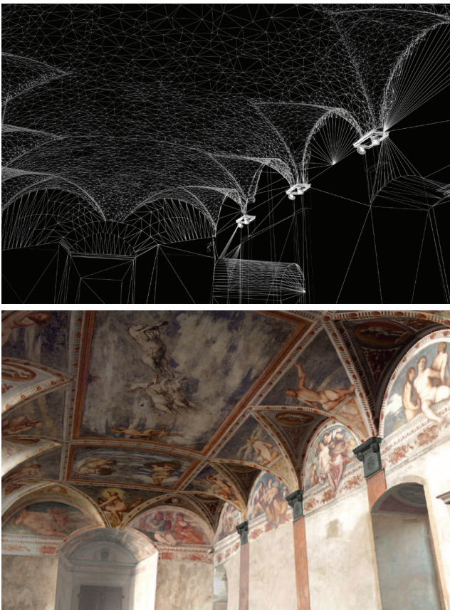
Figure 7: Wire-frame and textured model of the Romanino loggia vaults in the Buonconsiglio castle.
